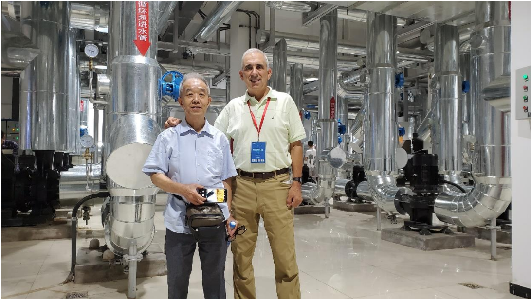
Immaculate mechanical room.
